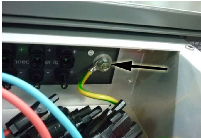
Fig. 30: Earthing of the ConnectionBox
