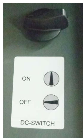
Fig. 27: DC Circuit Breaker
